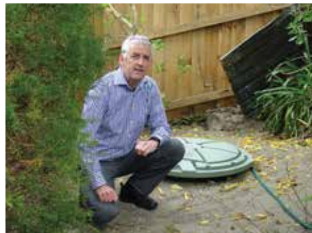
Mark Smith, of Rockinghorse Road, Southshore, had a pressure wastewater tank installed at the end of last year by SCIRT delivery team Fulton Hogan. Several hundred Southshore residents are getting the more reliable, easier to fix pressure wastewater systems in coming months
